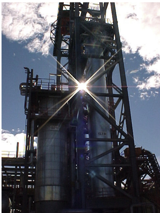
Fig. 13 – Ammonia loops at Arroyito HWP.
