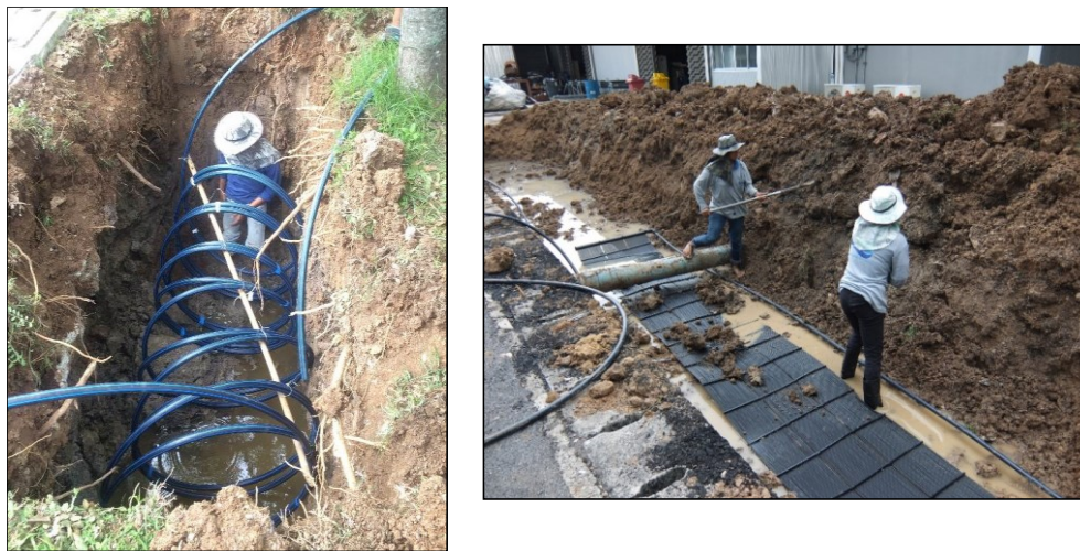
Figure 2. Installation of horizontal ground heat exchangers in Saraburi campus, Chulalongkorn University, Thailand.
