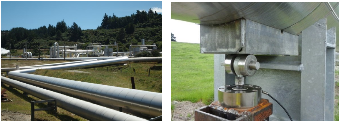
Figure 1: Pipes in steamfield on sliding pipe supports, and LC sensor installed at one such support.
