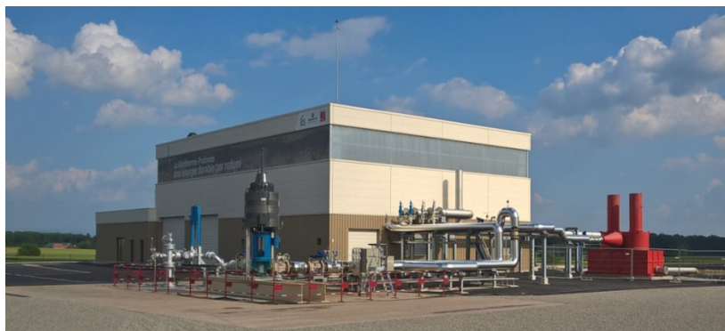
Figure 5: Rittershoffen geothermal plant. On the forefront, the production (right) and the reinjection well (left). The heat exchangers system is located inside the building.
