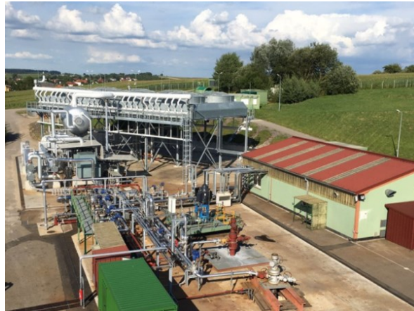
Figure 2: Geothermal plant of Soultz–EEIG Heat Mining, France.
