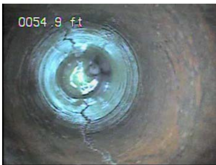
Figure 2. Borehole video log of a fracture created using controlled pressure fracturing (from SNL).
