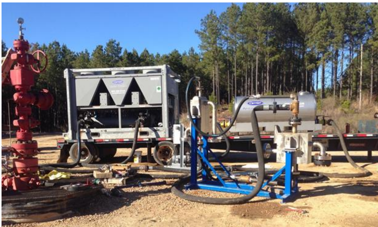
Figure 10. Two Heatric heat exchangers are located on the blue stand, with a 100 T chiller and surge tank in the background.
