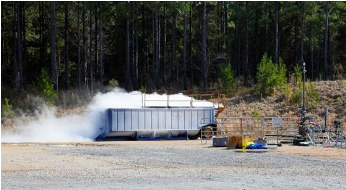
Figure 11. Venting operations from the F3 well into a “gas buster” equipped frac tank. The tank is designed to allow for dispersion of gas and collection of liquids during well venting operations.
