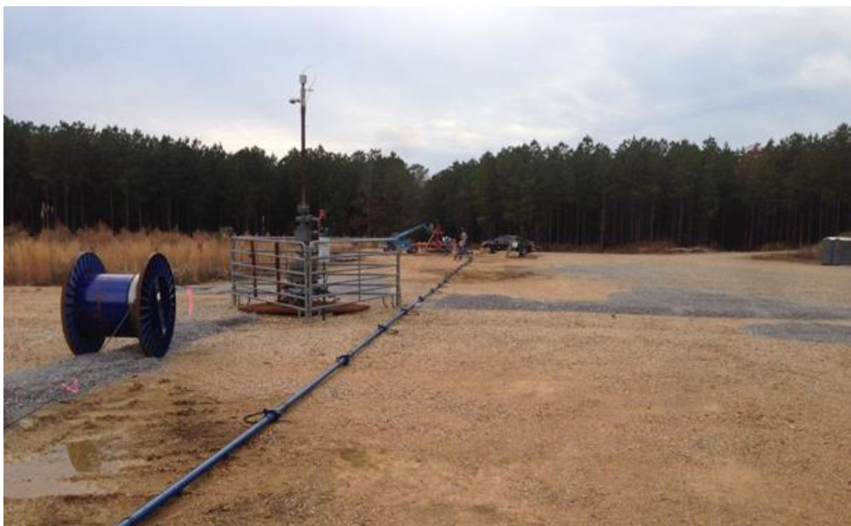
Figure 9. Flow iron looking toward F1 well from F3 well. This is the main recirculation loop for geothermally heated CO 2 . The F2 wellhead appears in the foreground with the more distant F1 wellhead painted red beyond it.
