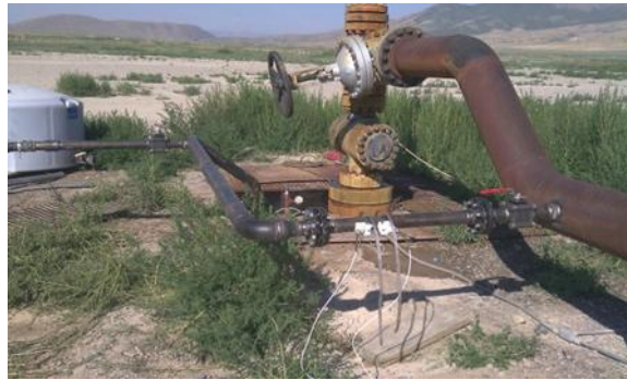
Figure 5: Pipeline sending injectate from 10” injection line into side outlet of RRG-9 with ultrasonic flow meter transducers mounted on 3” pipe.
