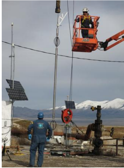
Figure 8: Sandia National Labs supervising Tiger Wireline in preparation for conducting a borehole televiewer survey of RRG-9.
