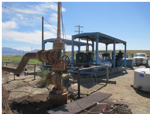
Figure 6: HP-165m plunger pumps installed next to RRG-9 to increase pressure of injection stimulation.
