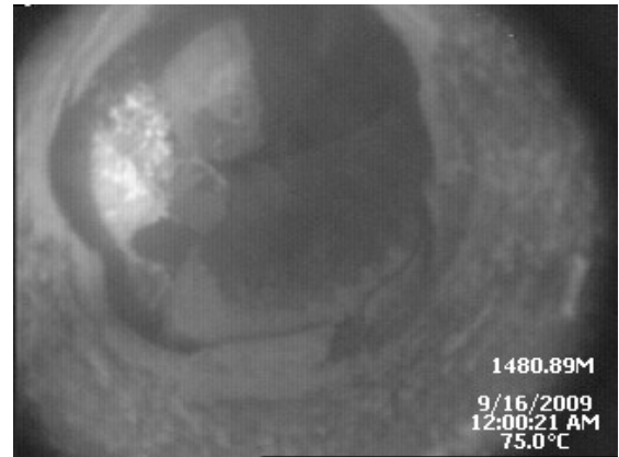
Figure 5: Liner damage found
