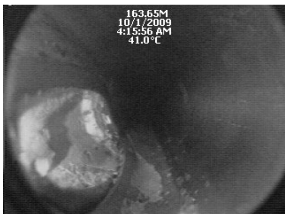
Figure 6: Down view image of the shallow casing damage
