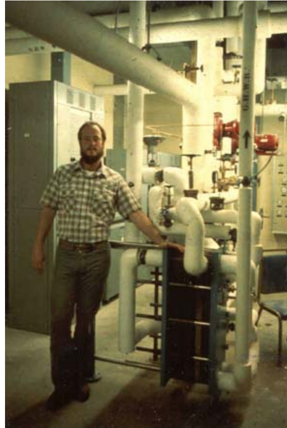
Figure 4: Plate heat exchanger in the College Union building.
