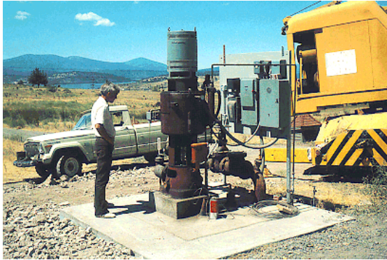
Figure 3: Gene Culver at well #6 showing the 75 hp (56 kW) motor and fluid coupling drive. The well house is moved for maintenance.
