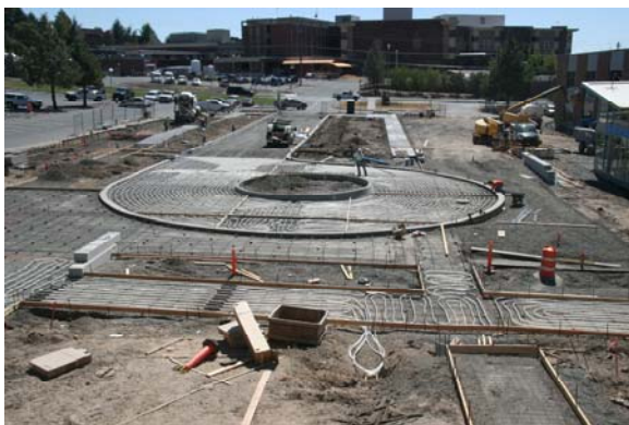
Figure 6: Installation of PEX pipe for the campus entrance snow melting system in 2008
