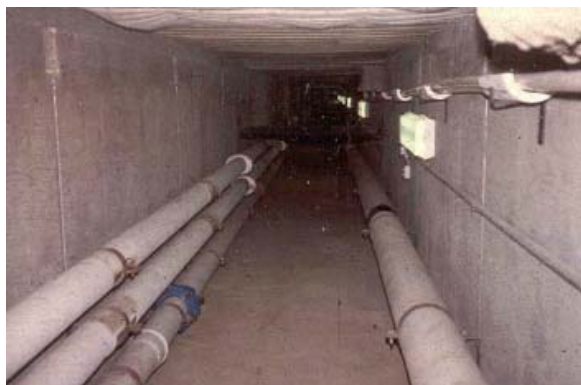
Figure 5: OIT utility tunnel with geothermal pipe and other utilities.
