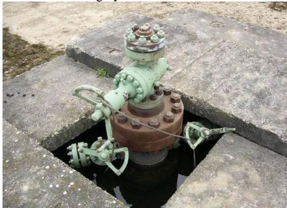
Figure 3: Head of an abandoned well in the Pannonian Basin.
