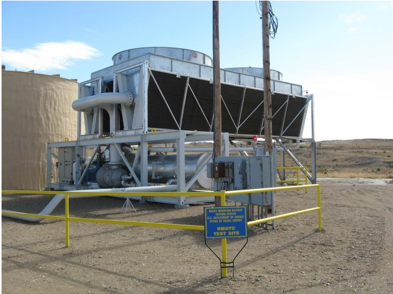
Figure 3: 250 kW ORC Low-Temperature Geothermal System at NPR-3
