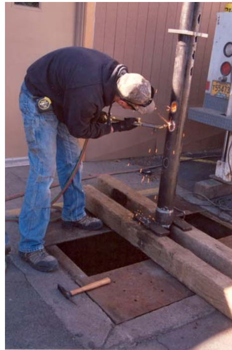
Figure 11: Cutting the 1-in diameter perforations in the promoter pipe for System Three.
