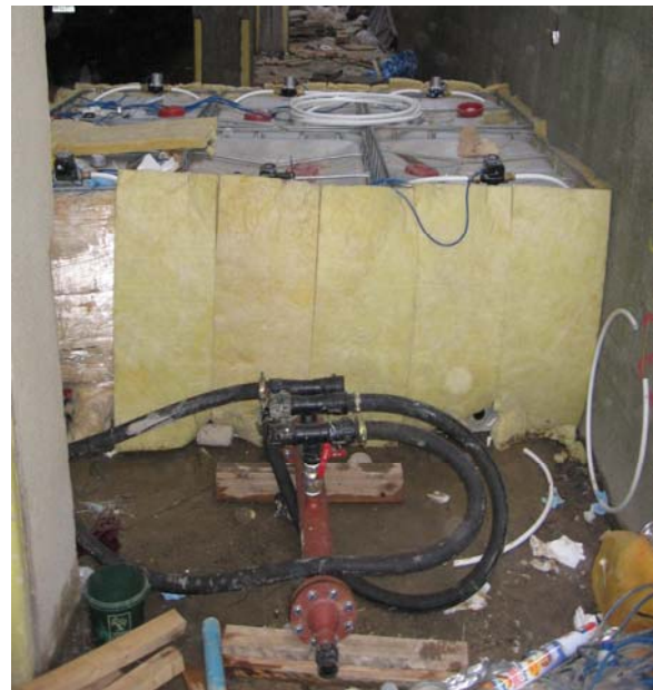
Figure 2. Plastic insulated containers for heated water storage
