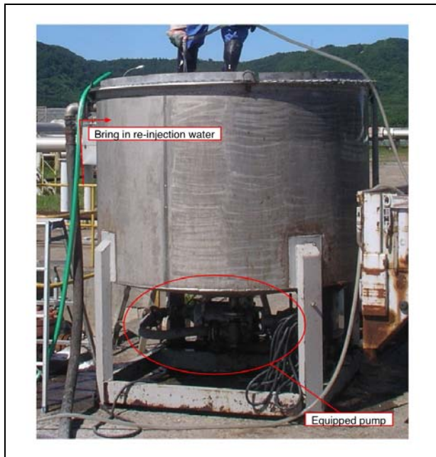
Figure 3. Photograph of the tracer mixer tank used in the Mori geothermal field. The tank is 3 kl in volume and equipped with a pump for mixing and injecting the tracer solution.
