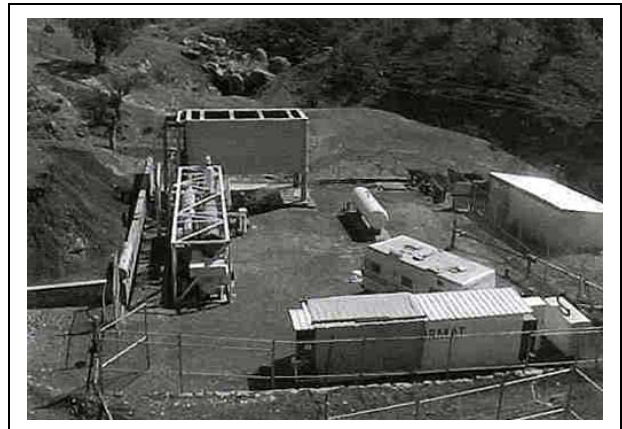
Figure 20. 300 kW binary plant at Maguarichic, Mexico.
