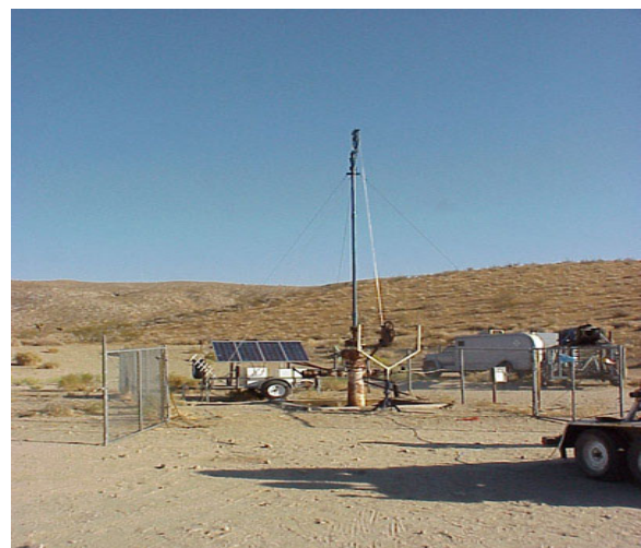
Figure 5. A photo of the uphole reservoir monitoring system.
