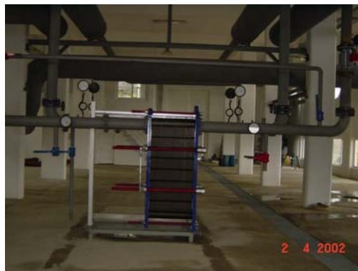
Figure 1: Salihli Geothermal Heating Center
