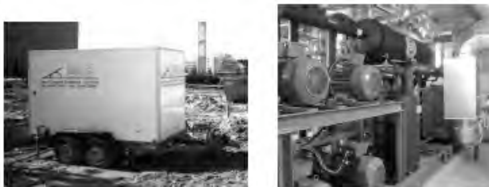
Fig. 15: left: Thermal Response Test equipment on site in Langen right: Heat pump in DFS-headquarters, Langen; to the left four motors driving the compressors. in the background and above evaporator and condenser.
