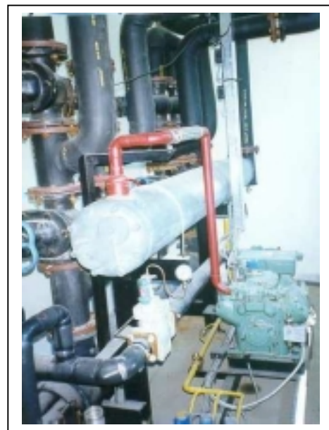
Figure 4. Heat pump (Curtis-Balkan Ltd, Sofia City)
