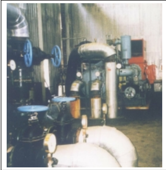
Figure 1. Heat pumps installation in "St. Konstantin and Elena" resort, (Northern Black Sea coast)
