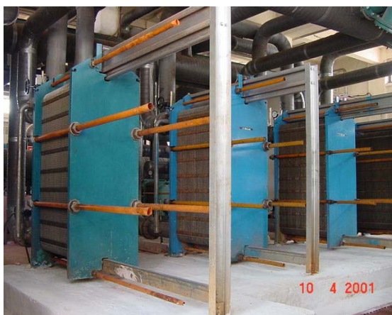
Figure 2: Kirsehir geothermal district heating center
