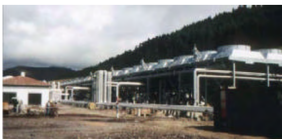
Figure 12: Ribeira Grande Binary Plant.
