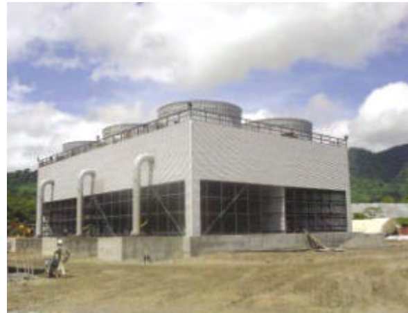
Figure 10: Lihir Power Station.
