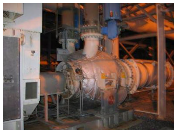
Figure 14: Salavatli Binary Plant.
