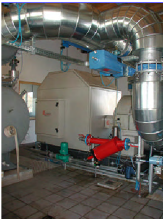
Figure 3: Altheim Binary Plant.
