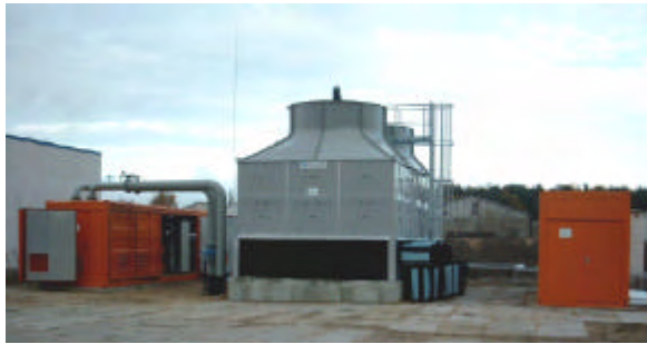
Figure 6: Neustadt Binary Plant.
