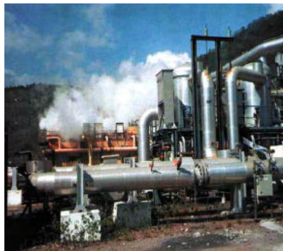
Figure 5: Bouillante Binary Plant.
