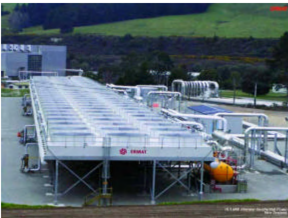
Figure 9: Wairakei Binary Plant.
