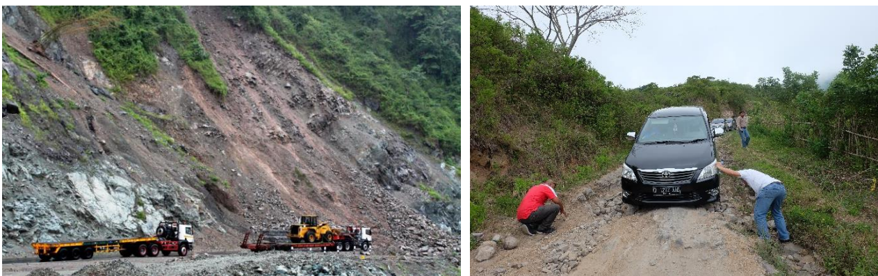
Figure 6: Access road conditions to one of the locations of geothermal prospects in eastern Indonesia that have the potential for landslides during rain and endanger road users (left) (Purba, 2018c; Purba, 2018d). Photo shows a car stuck in a road to a geothermal drilling location in one of geothermal prospect areas in Eastern Indonesia (right).
