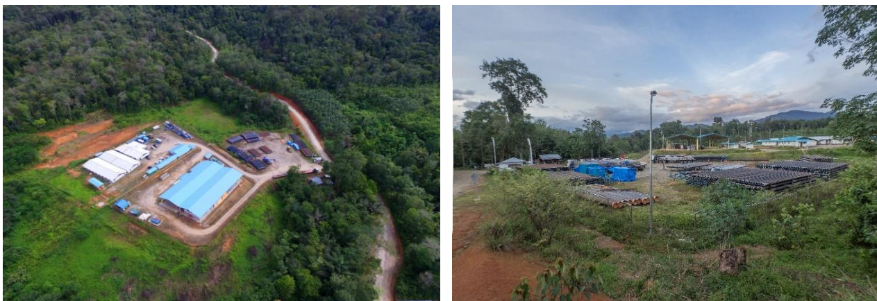
Figure 5: Photos of basecamp, warehouse, site office, and casing storage area in one of the geothermal exploration projects in Indonesia
