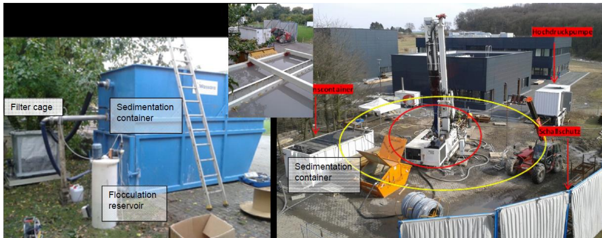
Figure 7: drill site (right) at GZB during DTH hammer drilling, first sedimentation container (white) always in use, second stage cleaning (optional) on left side including lamella cleaner and flocculant station.
