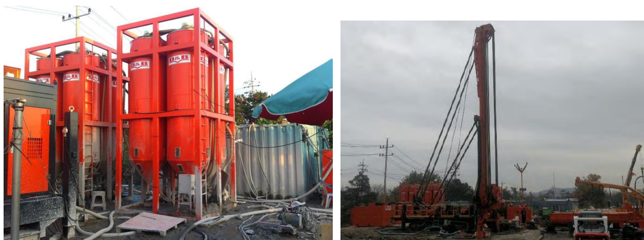
Figure 10: Test drill site in South Korea during DTH water hammer drilling down to 5.000 meters (right), drill mud treatment system for DTH mud hammer recirculation with sedimentation and lamella cleaning containers (left).
