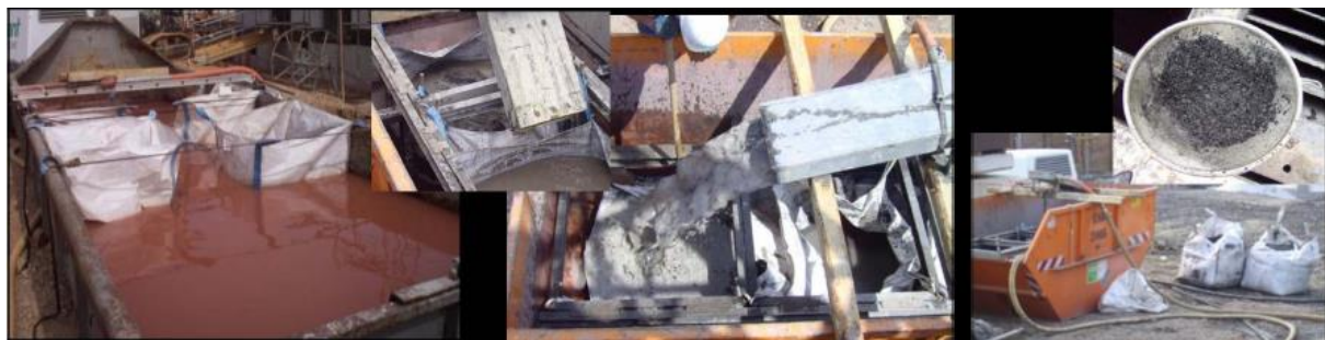
Figure 8: drill site at GZB during DTH hammer drilling : sedimentation container is lined and set up with commercial big packs for full recycling of drill cuttings; sample of cuttings and sacked material (right).
