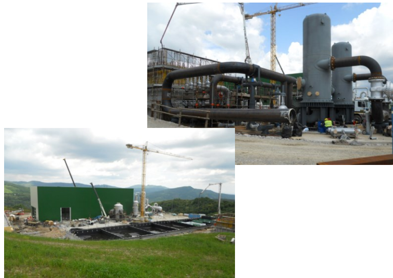
Figure 10: Bagnore 4 (40MW) power plant.
