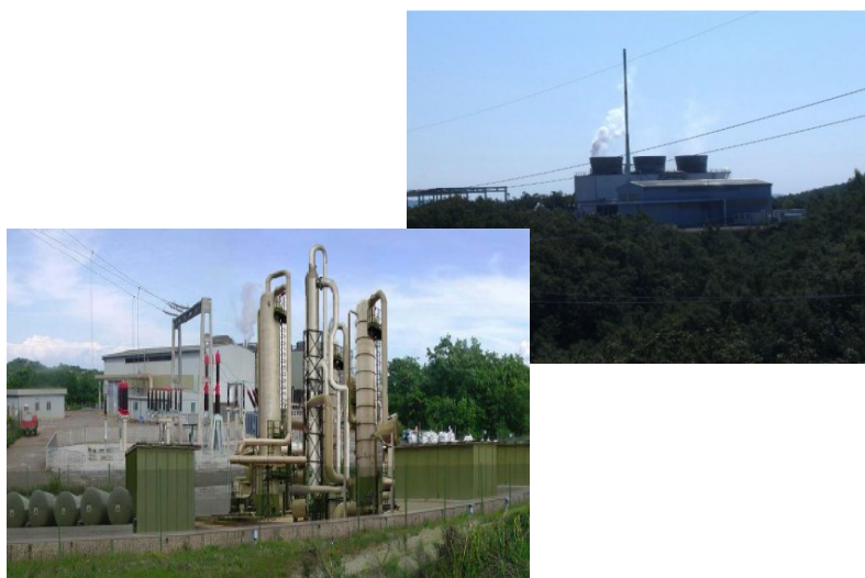
Figure 5: Rancia (20MW) and Rancia 2 (20MW) power plants.
