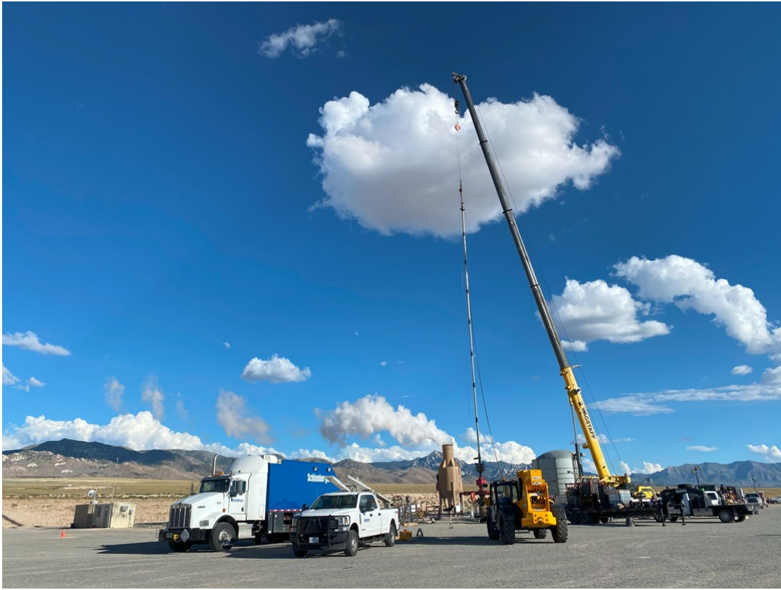
Figure 11: Utah FORGE Well 16B test site with lubricator stacks for chemical tool.
