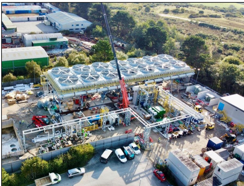
Figure 3: An aerial photograph of the United Downs Power Plant taken during the final stages of construction in Q4 2024.
