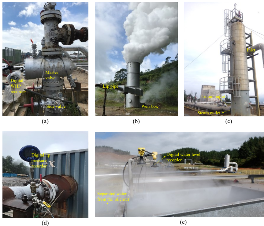
Figure 6. Photographs of production testing monitoring system facilities at (a) well head, (b) silencer, (c) separator, (d) lip pipe, and (e) weir box (taken by first Author).
