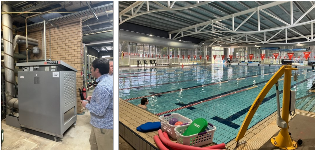
Figure 12: Existing gas burner for hydronic heating of the swimming pool and buildings at the BARC
