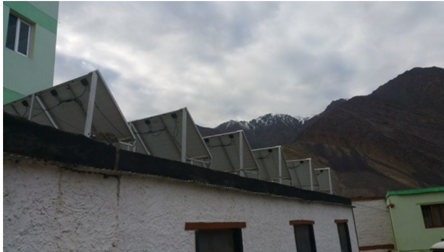
Figure 2. Solar panel fixed over the heating space for power required to run the electrical appliances for regulating hot water
