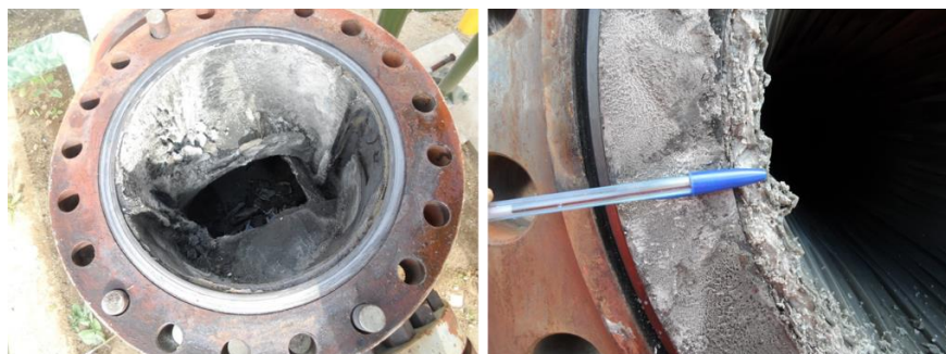
Figure 4: Photographs showing silica scaling, about 2 cm thick, at the two-phase line in OW38 in 2015.
