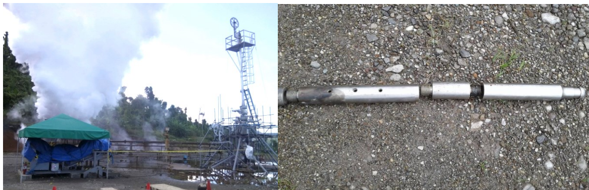
Figure 7 (Left Picture) Winch with the CTU set-up covered in tarpaulin to protect from inherent corrosiveness of geothermal fluids (left) and the well head set-up installed with the recovery spool for the injector head (right). (Right Picture) Injector head after the FMS test.
