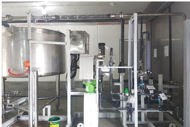
Figure 5: Stainless steel holding tank (left) and Pulsafeeder GLM series transfer pumps (right)
