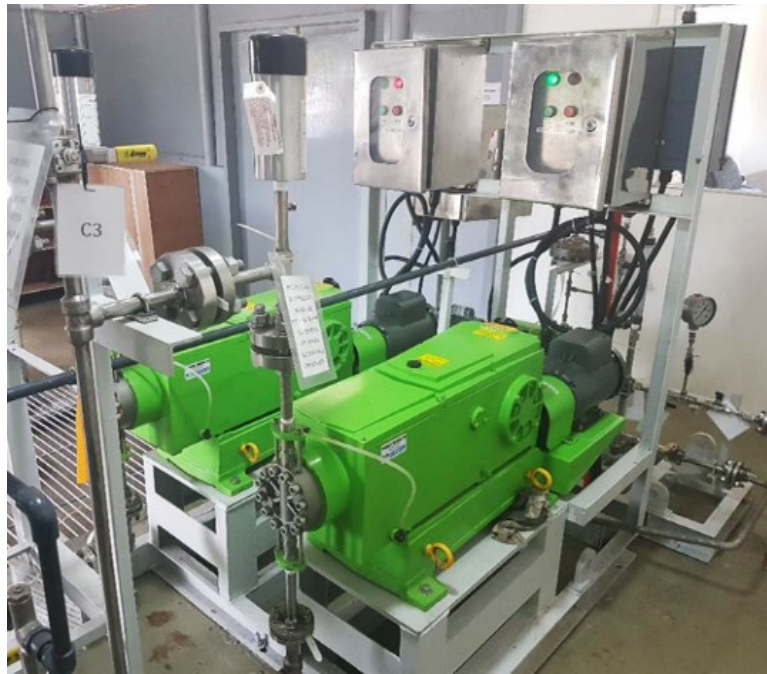
Figure 6: Pulsafeeder 7660-S-E used as injector pumps for the FMS. Two (2) units are installed to serve as a 100% back-up.
