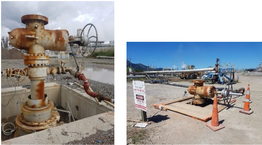
Figure 5: Before and after photos of KA47 wellhead lowering and master valve refit.
