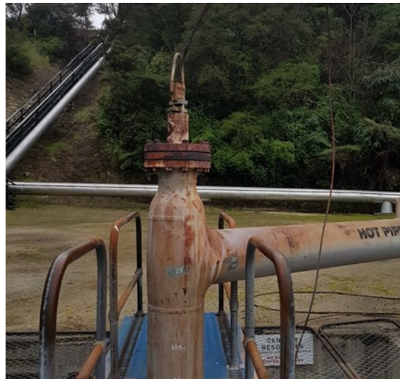
Figure 2: Production well with first-generation anti-scalant tube installed.
