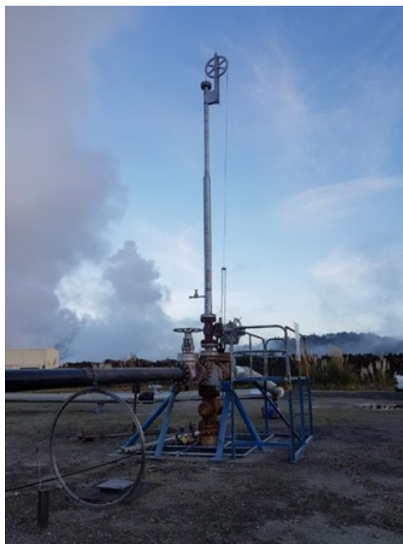
Figure 10: KA27 with new anti-scalant system installed.
