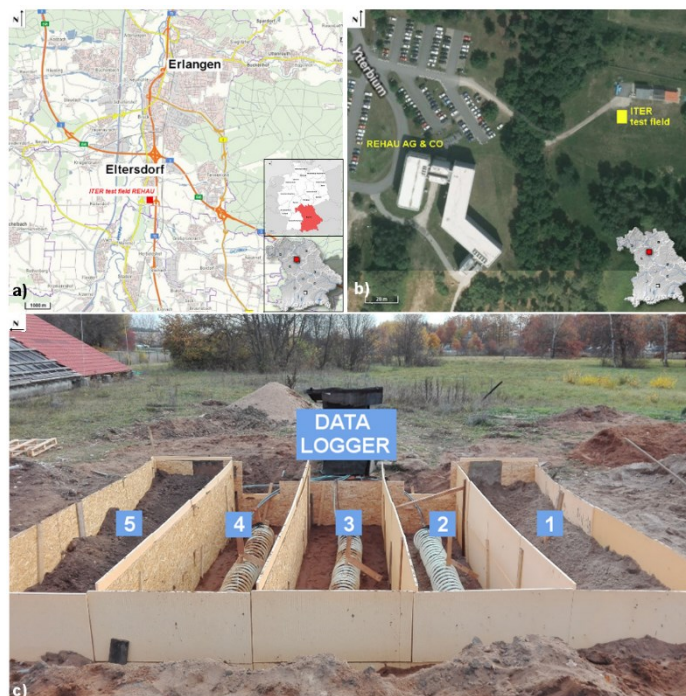
Figure 1: ITER Project test site location in Eltersdorf, Bavaria, Germany (a) and in the REHAU AG & Co facilities (b) [modified by Bayern Atlas]. Installation of 5 helix collectors in different sectors filled in with different soil mixtures and thermally isolated with XPD panels (c):
