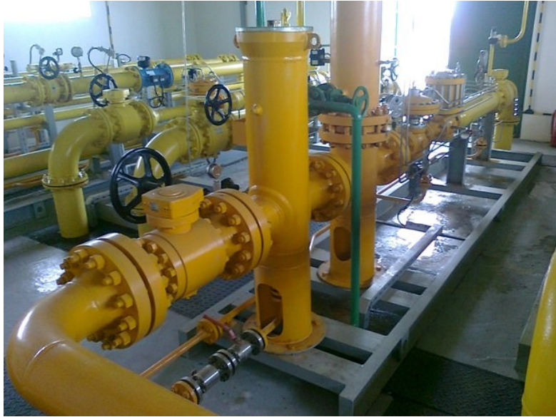
Figure 5: The Nagylengyel gas pressure reduction station
