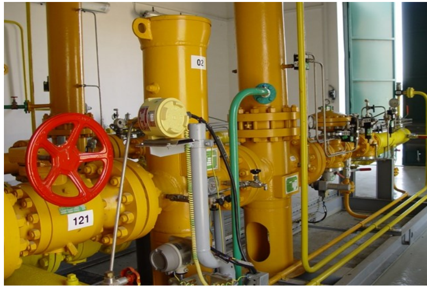
Figure 4: The Kőröshegy gas-pressure reduction station
