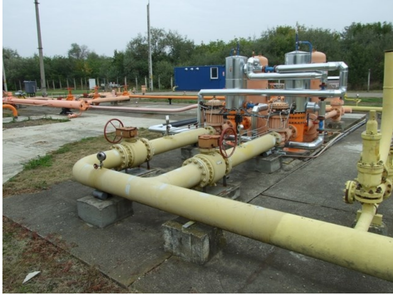
Figure 8: Szeged gas pressure reduction station
