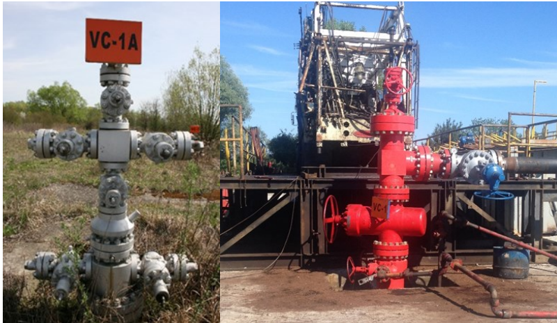
Figure 3: Christmas tree (left) and geothermal wellhead (right) of VC-1A well
