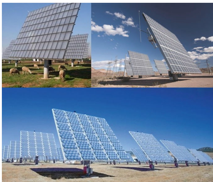
Figure 2. PV panels (Ritcher et al, 2012)
