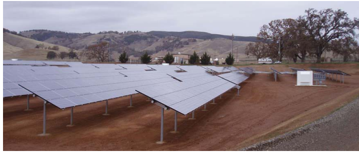
Figure 17: the PV system with the pump house (in back) for the Southeast Geysers Effluent Pipeline (Eney and Rudisill, 2009)
