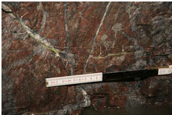
Figure 9: A close view of fracture 8, on the south side of ED4, at the lower and west end of the inclined structure as it leaves the structure to become nearly horizontal again.
