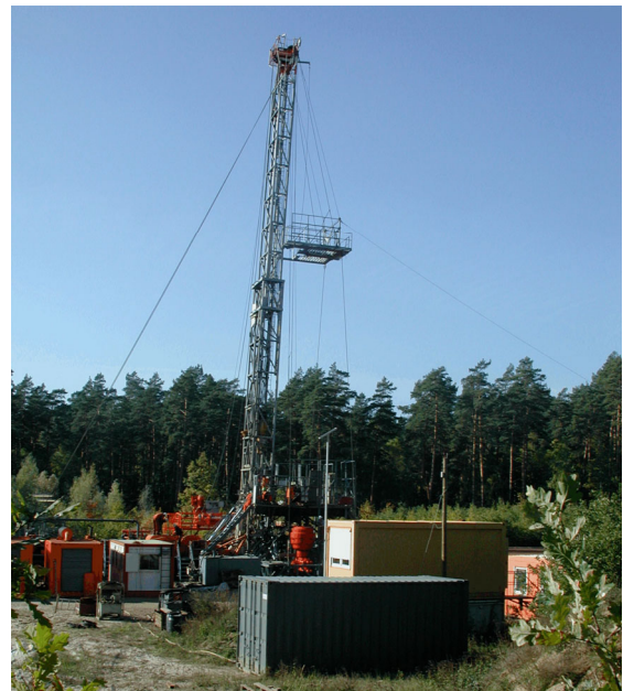
Figure 1.: Drilling rig for the opening and clearance of the borehole, Groß Schönebeck, October 2003
