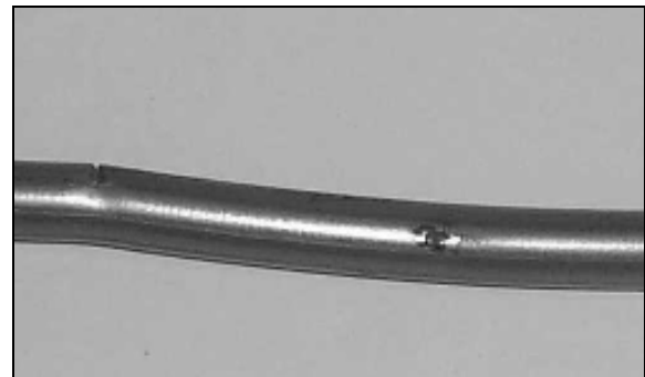
Figure 2. Closer view of the opened cracks which penetrated the tubing and the pits with associated corrosion products.
