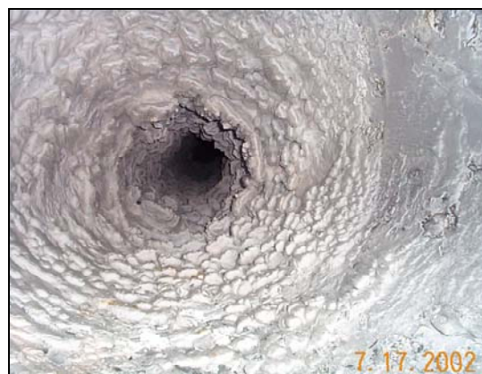
Figure 6. Section of 508 mm two-phase line 179, 2m downstream of ell OK-2 tapping
