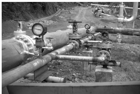
Figure 3. The CO 2 injection piping set-up near well 1R8D branchline.
