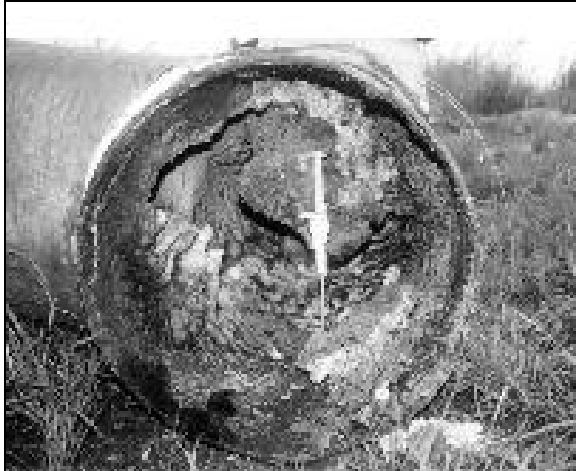
Figure 5. The 610-mm diameter header where fluids of OP-5DA and OP-6D mix. The main blockage area.
