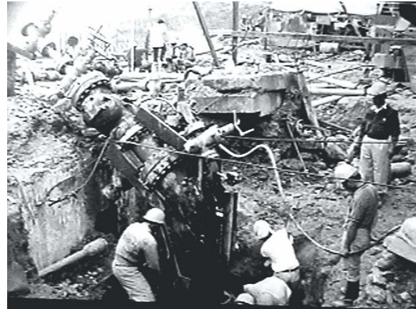
Figure 2. The damage on the wellhead of OK 5.
