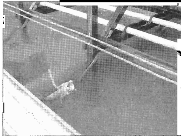
Figure 5. Vacuum separator discharge at the cooling tower basin.
