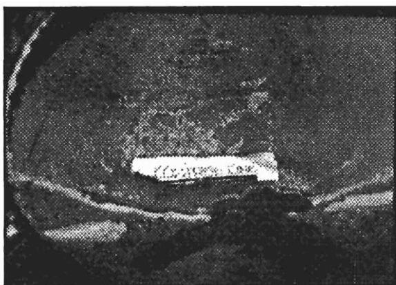
Figure 3. Untreated retention vessel
