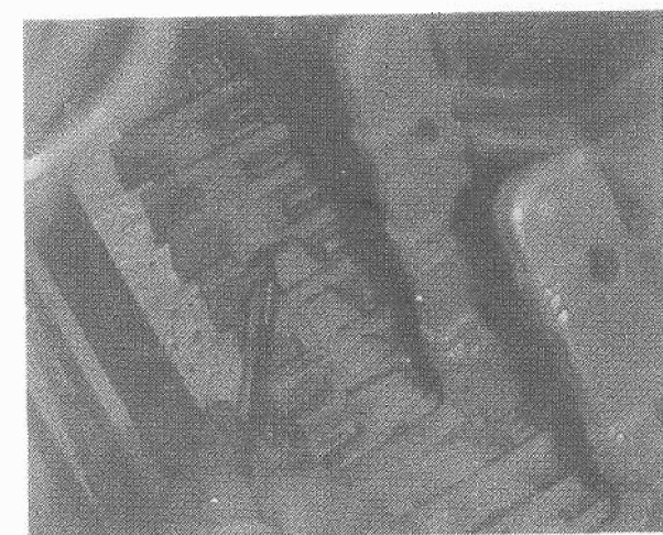
Figure 6b. Unit 1 exciter coil-end showing the presence of copper sulfide (CuS) black deposits.
