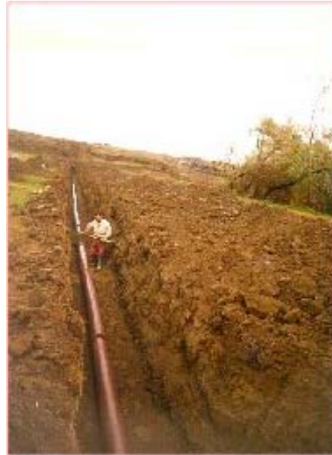
Figure 3: Pre-Insulated FRP pipes for geothermal water transportation
