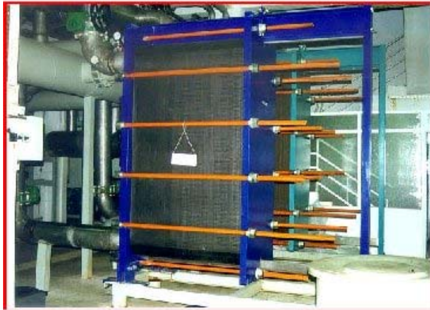
Figure 1: Plate type heat exchangers used in Izmir Balcova Geothermal District Heating System
